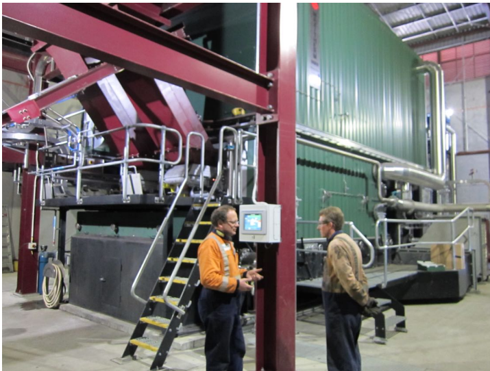
14MW coal fired boiler - Timaru
