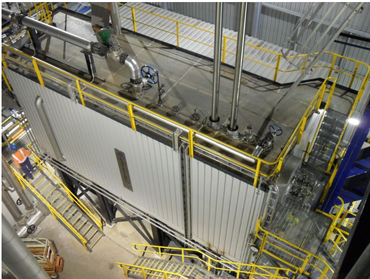
15MW coal fired boiler - Invercargill
